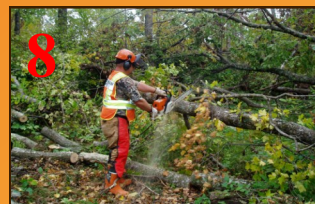
8 Remove dead branches, trees and shrubs within 100 feet of structures.
