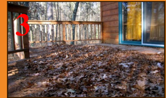
3 Clean areas that tend to be natural traps for debris (decks, window wells, around foundation).
