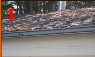
1 Remove pine needles, leaves and branches off roofs and out of rain gutters.
